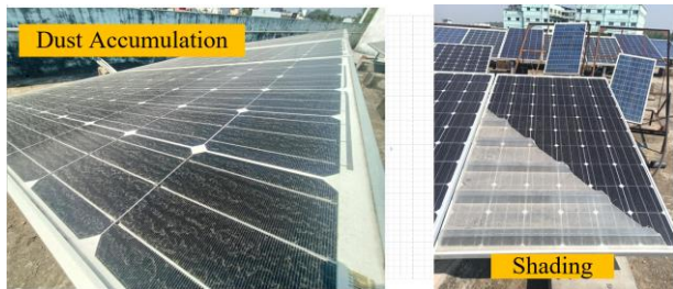
Figure 32. Fault creation on PV panels
