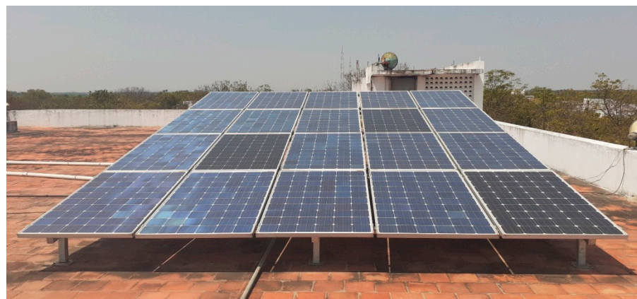
Figure 4. 5 kW PV Array.
